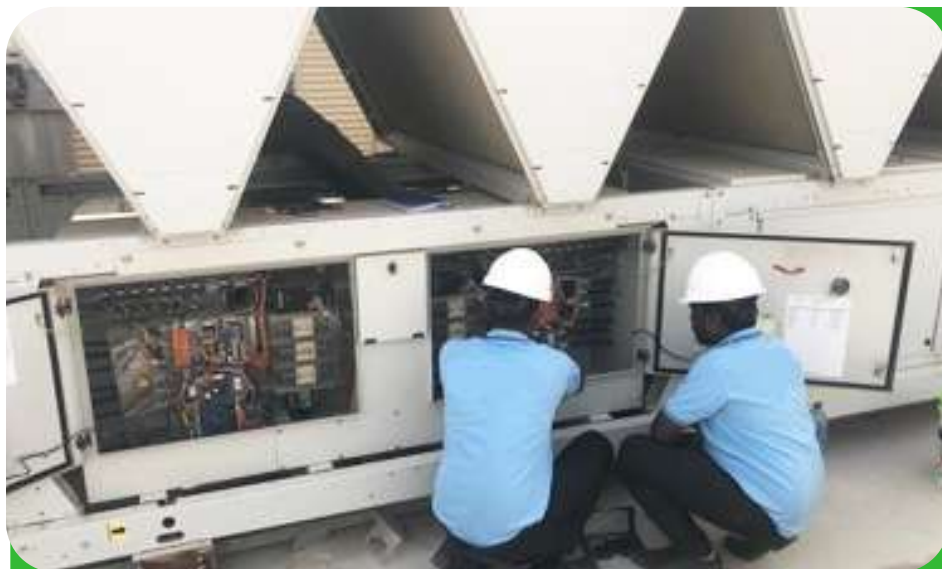
> Chiller Maintenance & Troubleshooting
