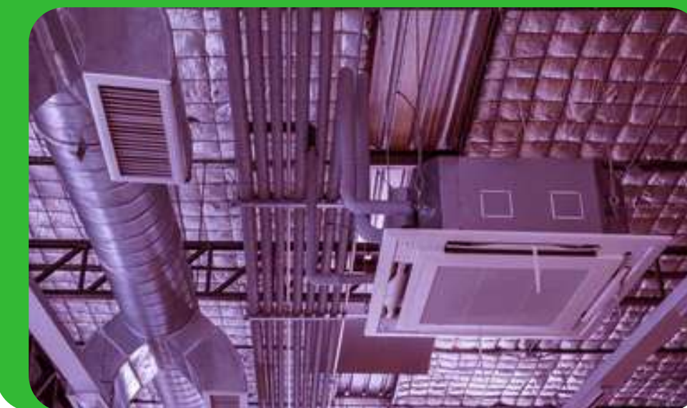
> HVAC Systems & Maintenance Services
