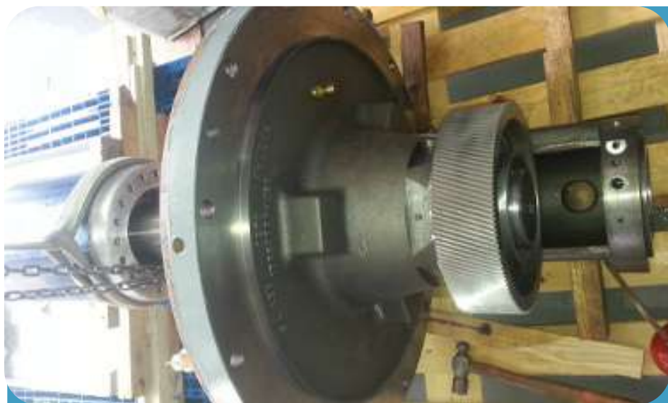
> Centrifugal Chiller Services
