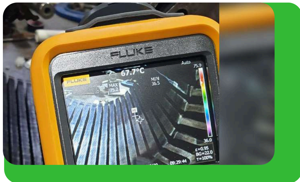
> Chiller Thermography Testing
